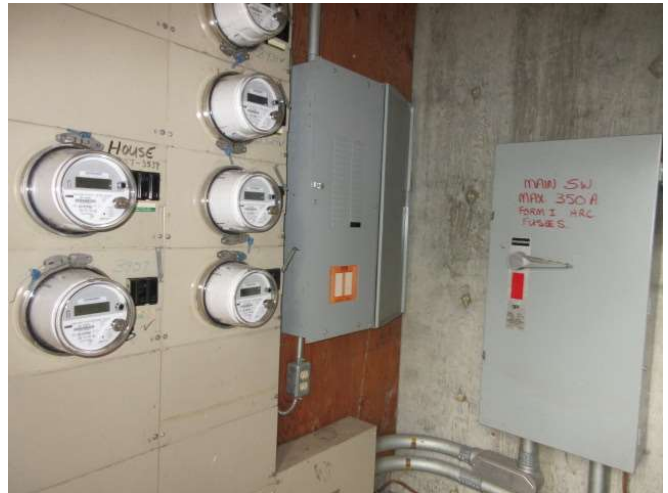
Photo 20: Typical electrical room.
