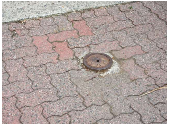
Photo 18: Typical water shut-off from the main supply line.
