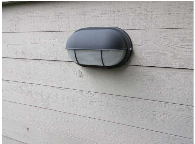
Photo 21: Typical new lighting installed at the walkway along Arbutus Street.
