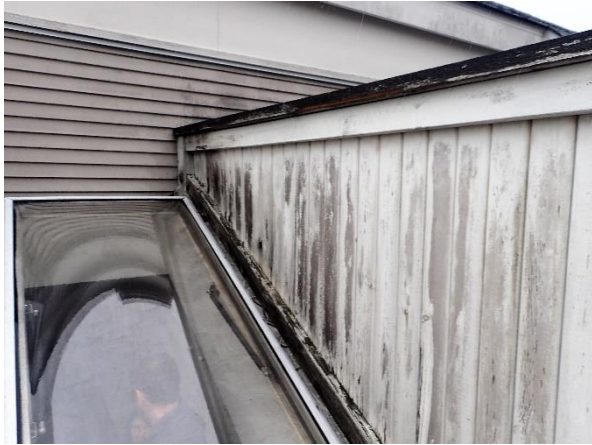
Photo 2: Sample of fade paint finishing, and decayed elements noted on fencing on the roof decks.
