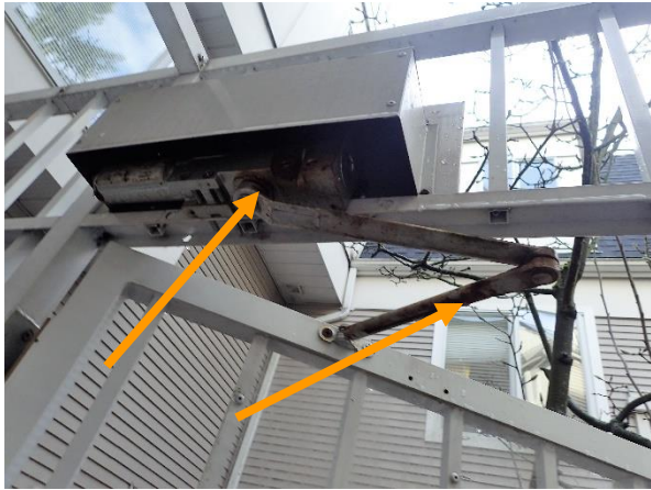
Photo 1: Corrosion observed on some elements of door control mechanism of a few entry gates.
