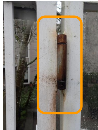
Photo 2: Corroded hinges noted at multiple locations.
