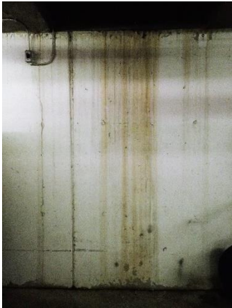
Photo 3: Staining noted on the concrete foundation wall at Stall #57 behind the parkade exhaust fan. Remove staining and monitor if reoccurs, repair as required.
