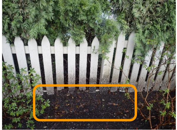
Photo 2: Gothic Picket Fences installed at front side of the property. A sample of damaged fencing at front side of the complex.
