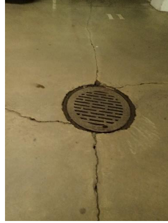
Photo 2: Noticeable cracks observed in slab on grade around the drainage that need to be repaired.
