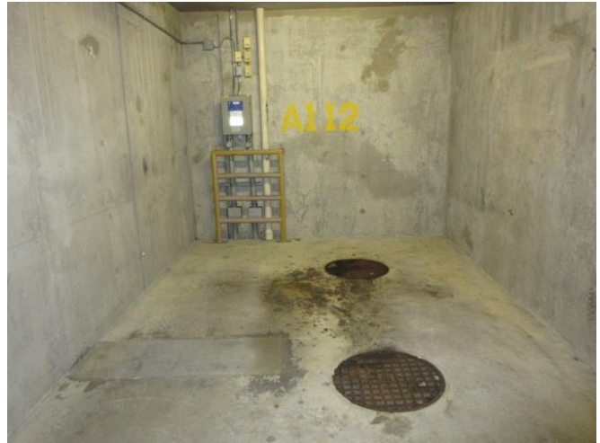
Photo 20: Typical storm sump controls.
