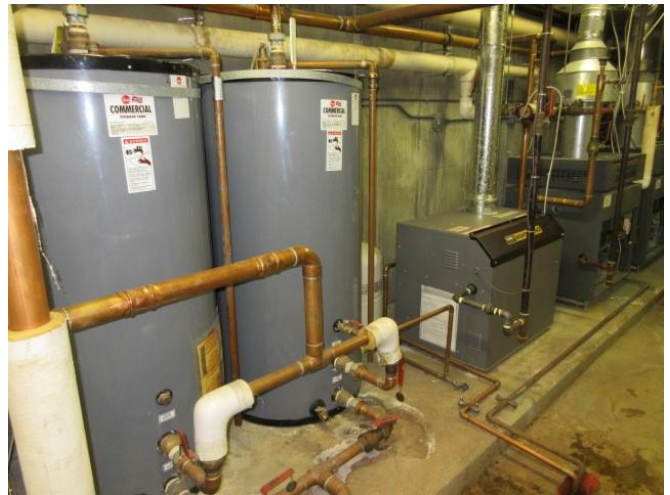
Photo 18: Typical domestic hot water boilers and storage tanks.
