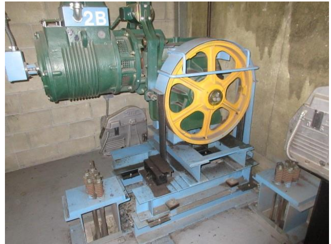
Photo 23: Typical elevator machine.
