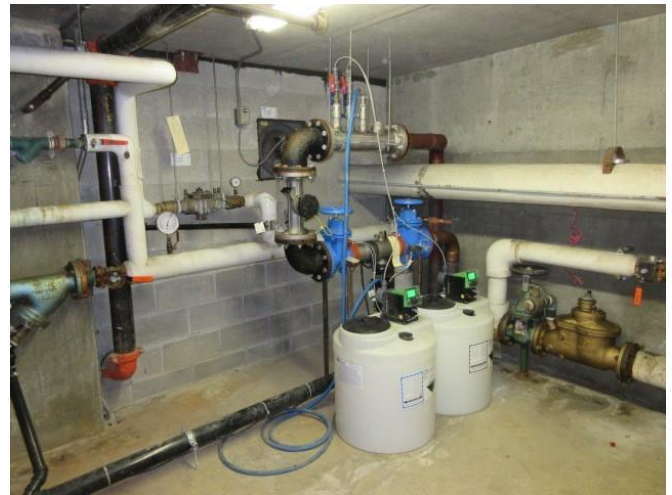
Photo 19: Domestic water and Hytec equipment.
