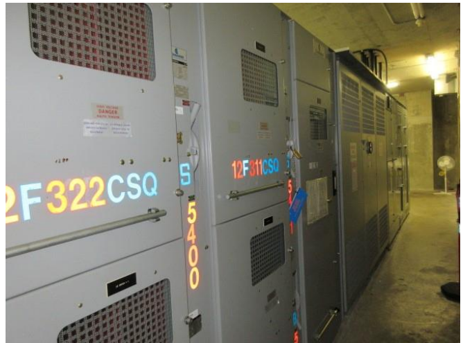
Photo 21: Main electrical equipment.
