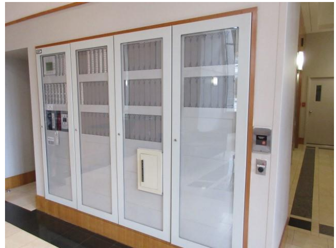
Photo 11: Fire alarm control panel.
