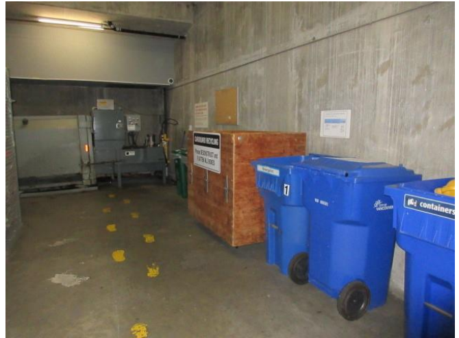
Photo 24: Garbage room with compactor and recycle bins.
