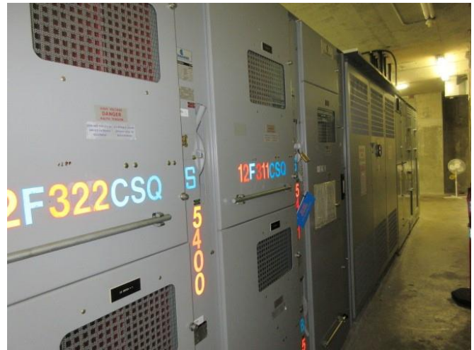
Photo 21: Main electrical equipment.
