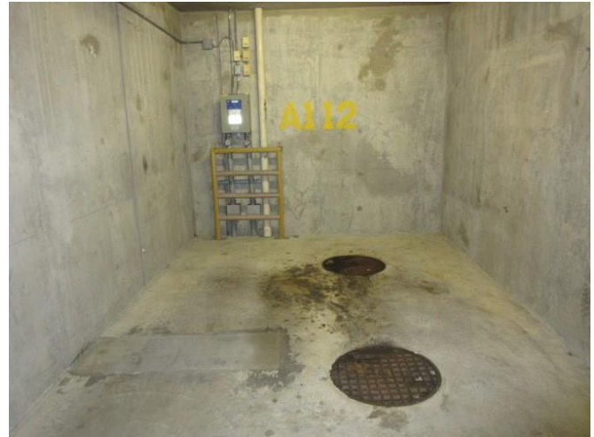
Photo 20: Typical storm sump controls.
