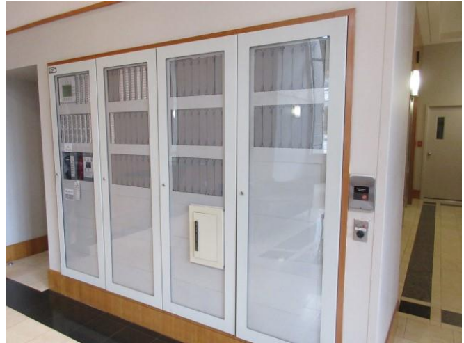
Photo 11: Fire alarm control panel.
