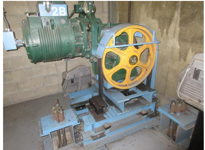
Photo 23: Typical elevator machine.
