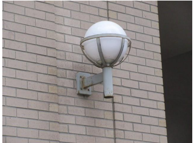
Photo 22: Typical exterior lighting.
