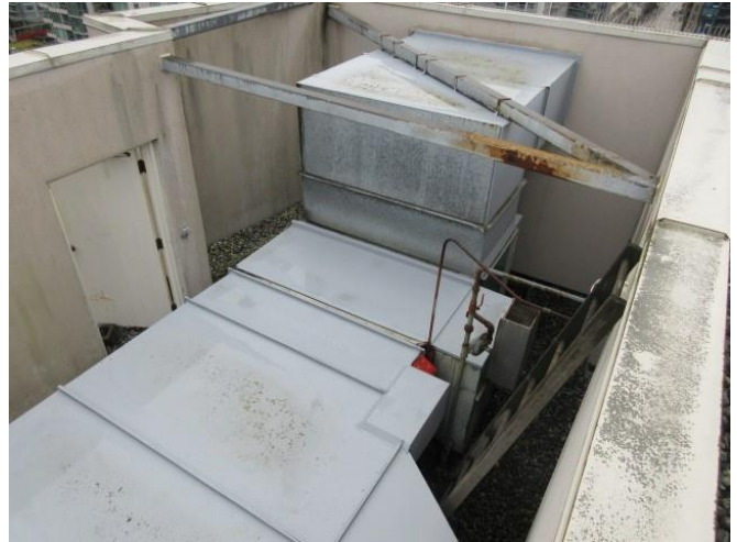
Photo 16: Roof-top make up air unit.
