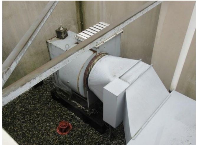
Photo 17: Smoke exhaust fan.
