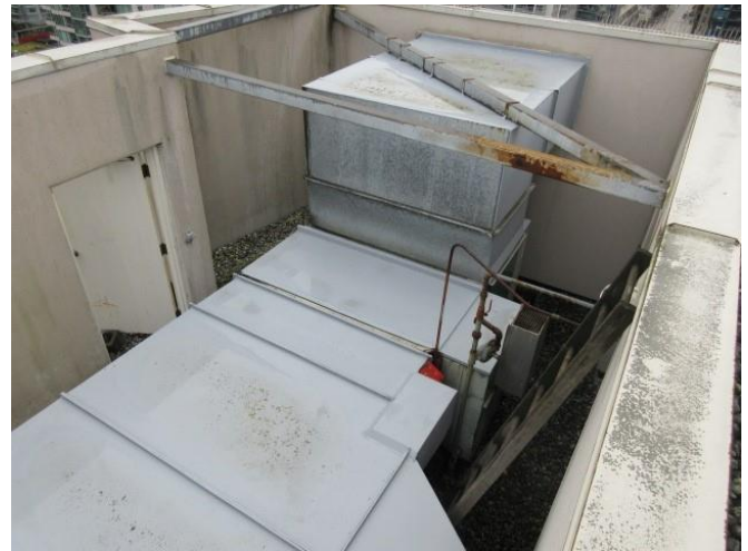
Photo 16: Roof-top make up air unit.
