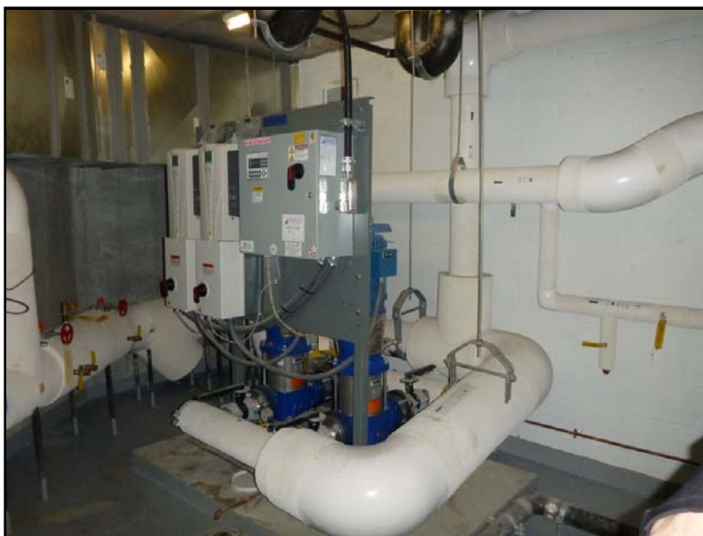
Photo No. 26: Main domestic water service and booster pumps
