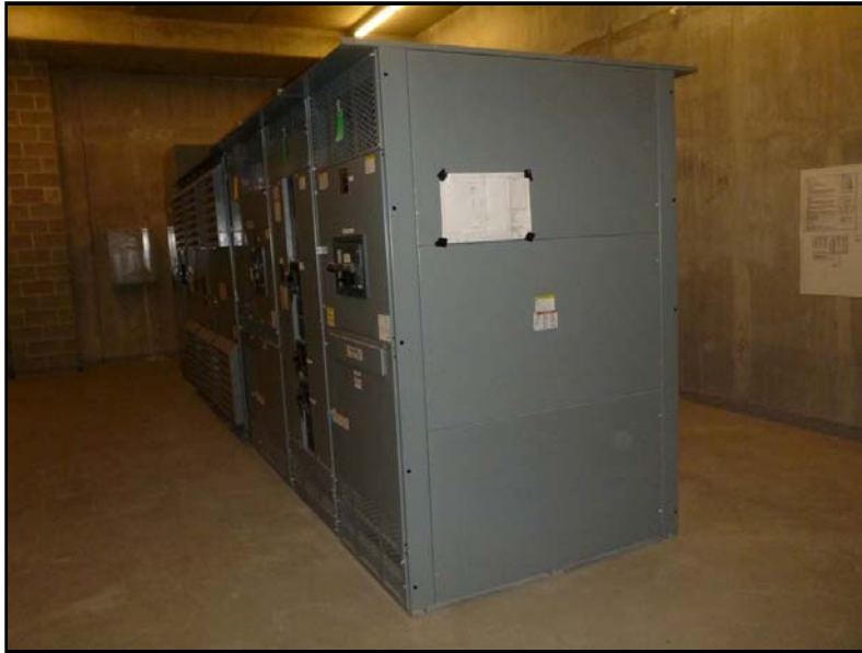
Photo No. 29: Electrical substation
