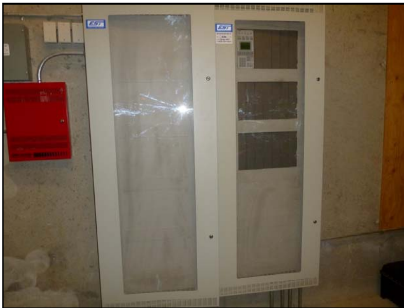
Photo No. 10: Fire alarm control panel
