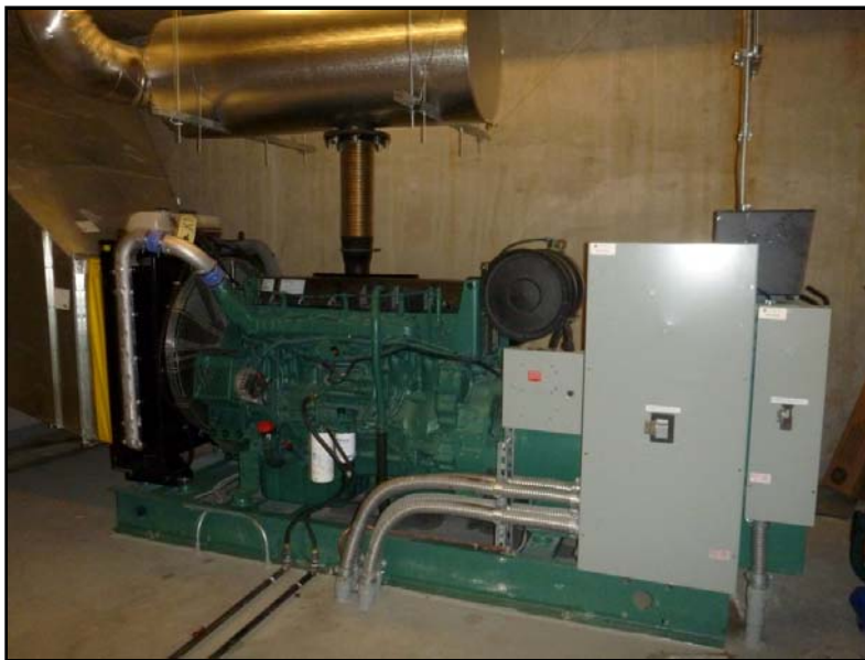
Photo No. 14: Emergency generator
