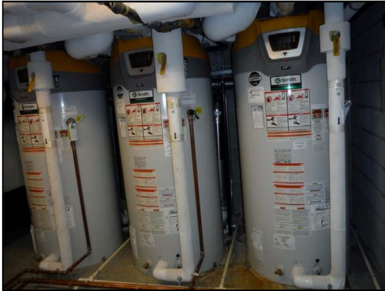
Photo No. 27: Domestic water boilers
