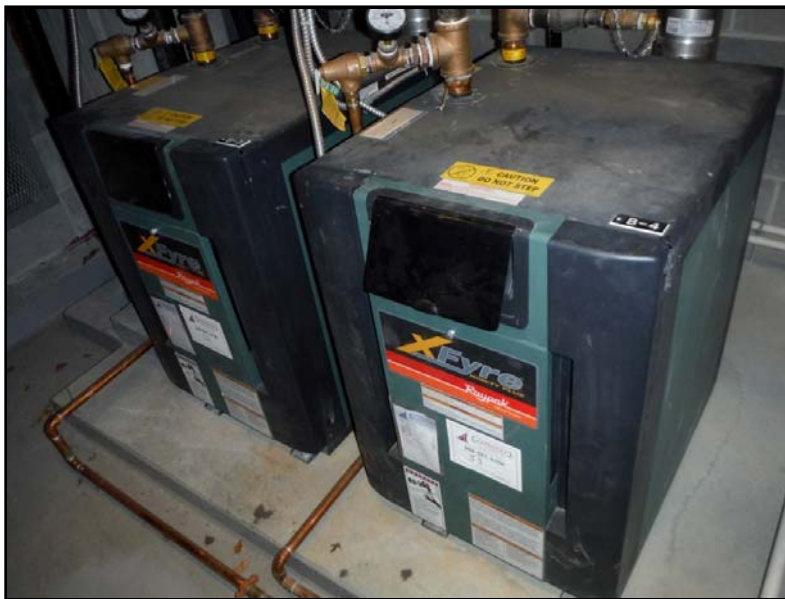
Photo No. 24: Heat pump loop boilers
