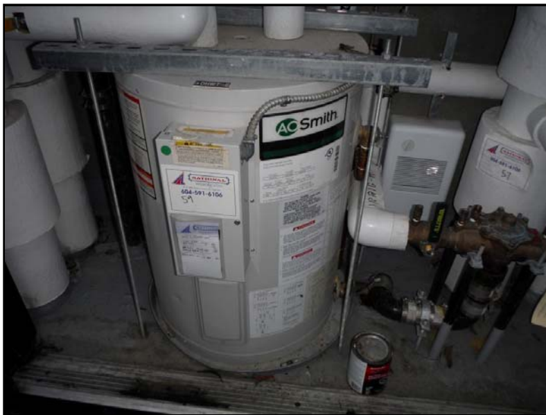
Photo No. 28: Typical domestic water re-heat tank
