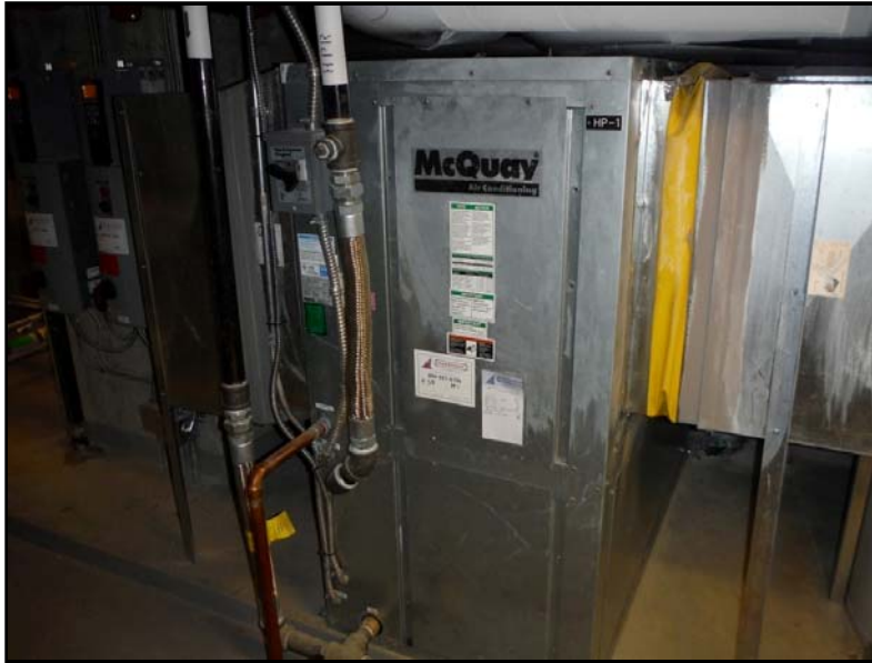
Photo No. 23: Transformer room heat pump
