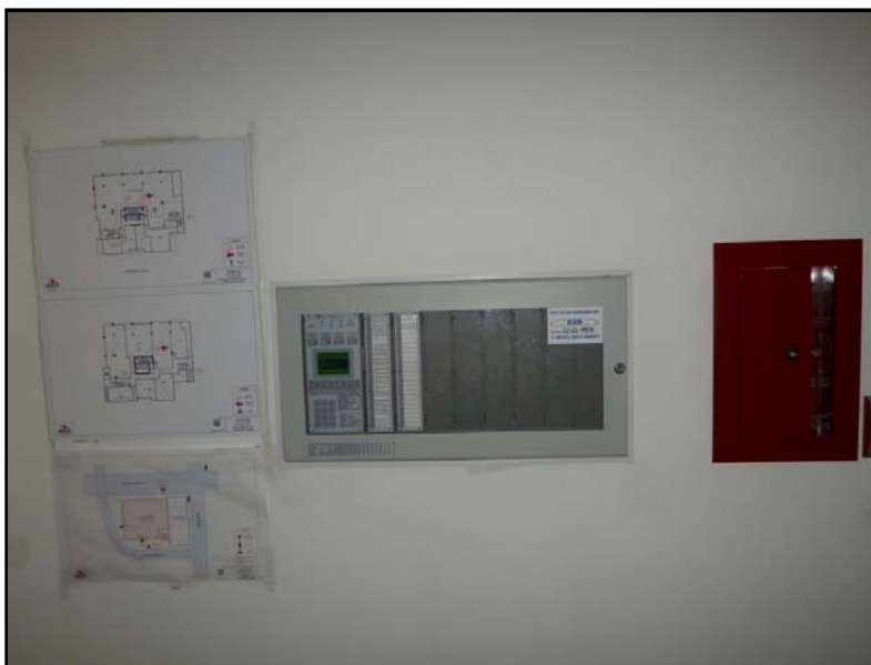
Photo No. 12: Commercial fire alarm annunciator panel
