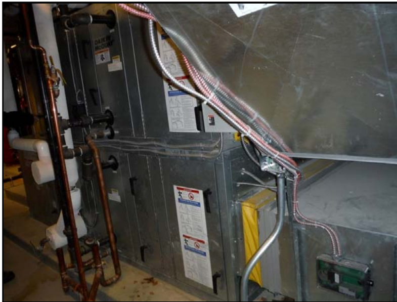
Photo No. 25: Heat recovery ventilator
