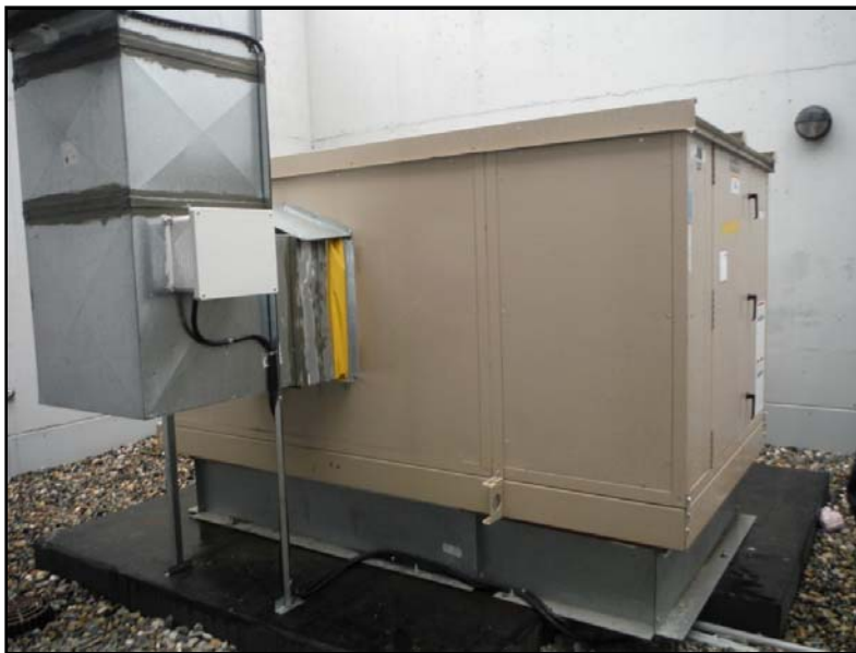
Photo No. 22: Make-up air unit
