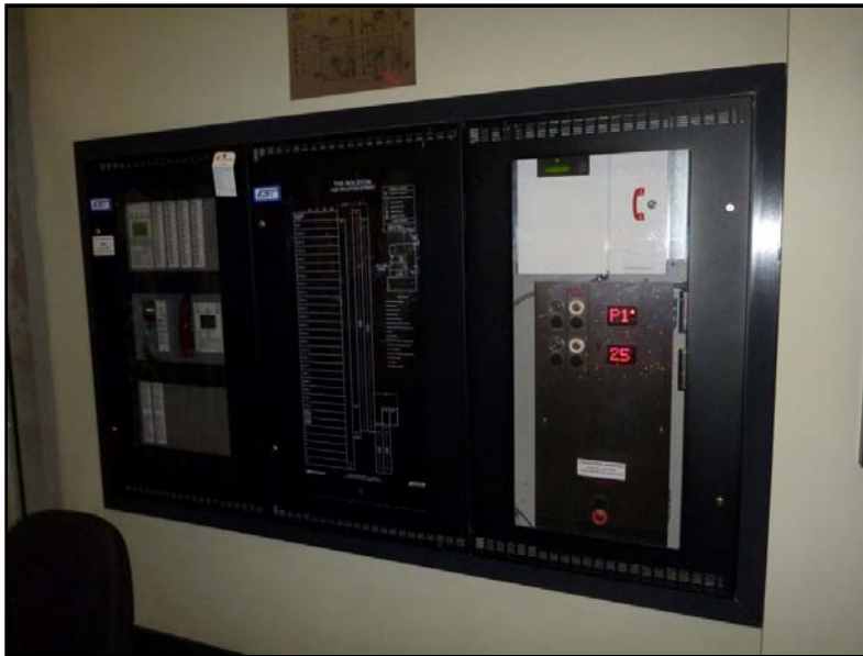
Photo No. 11: Residential fire alarm annunciator panel
