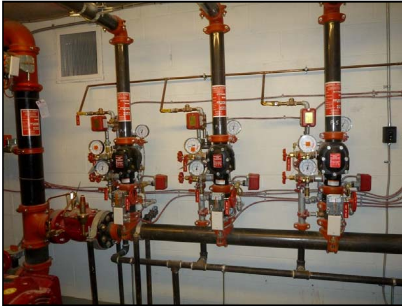
Photo No. 13: Main fire suppression service
