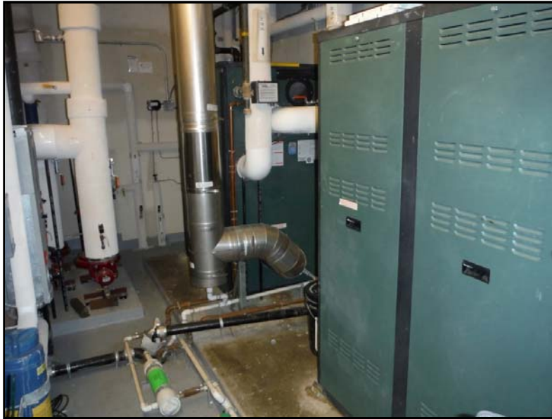
Photo No. 21: Central heating equipment
