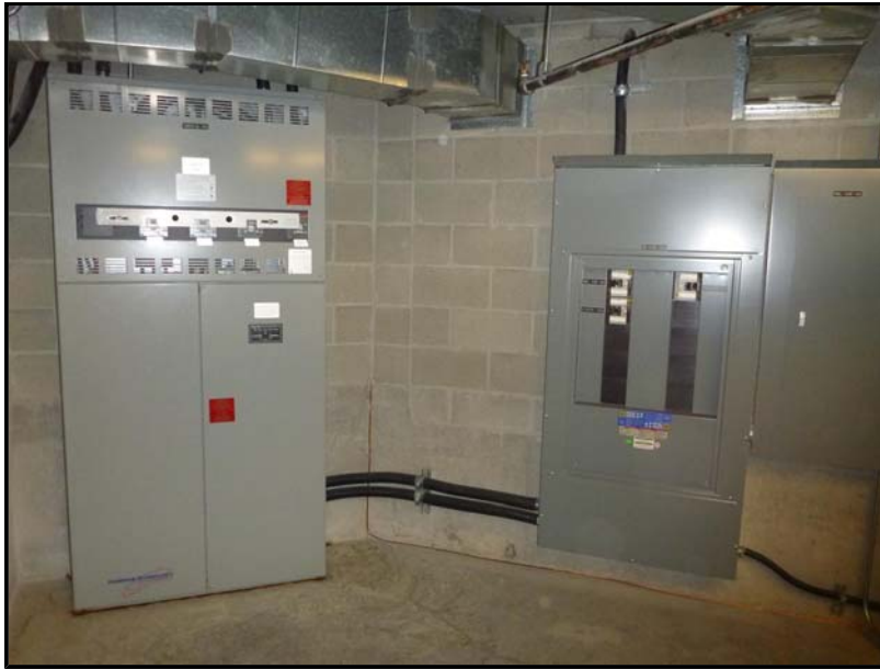
Photo No. 11: Automatic transfer switch and emergency distribution panels
