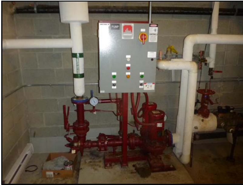
Photo No. 17: Booster pumps
