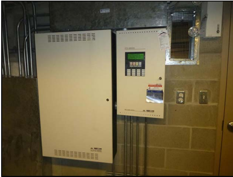
Photo No. 9: Fire alarm panel
