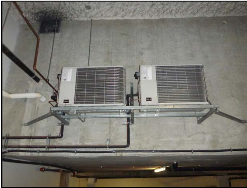
Photo No. 15: Air conditioning unit condensers
