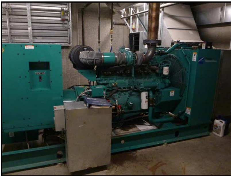
Photo No. 10: Generator
