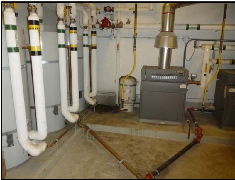
Photo No. 16: Domestic hot water boilers and storage tanks
