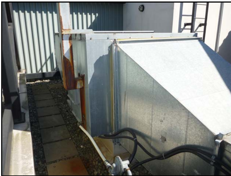
Photo No. 14: Make-up air unit
