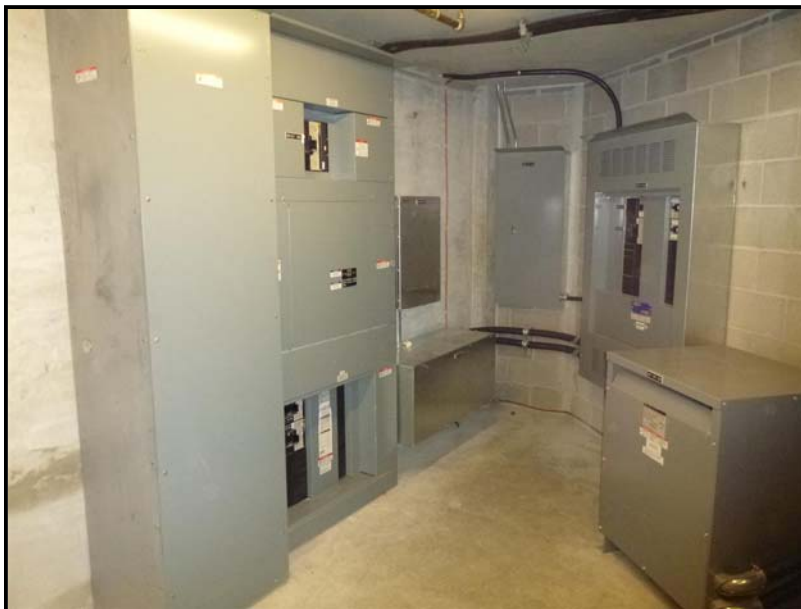
Photo No. 18: Main electrical equipment
