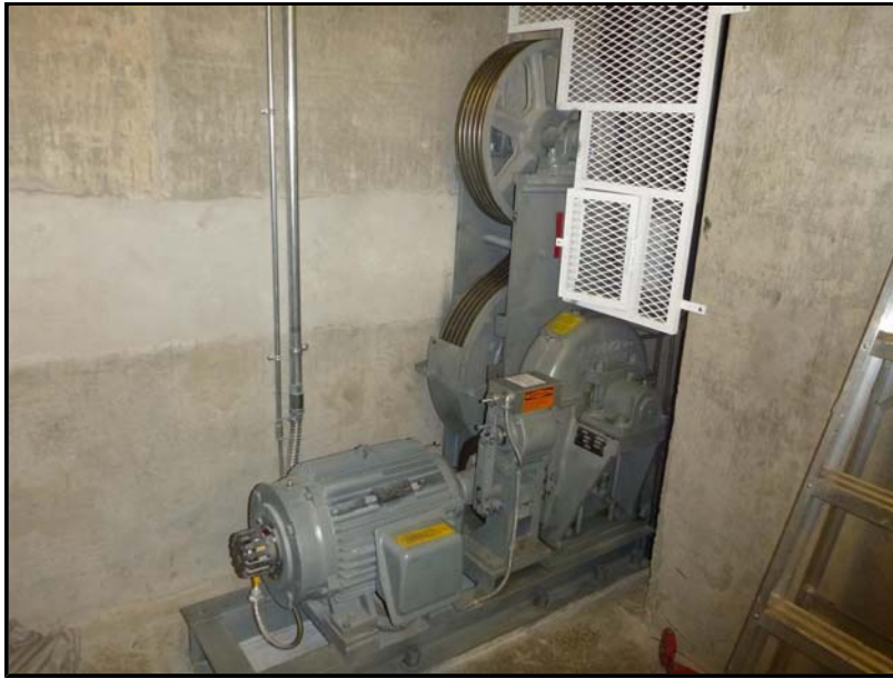
Photo No. 19: Elevator machine
